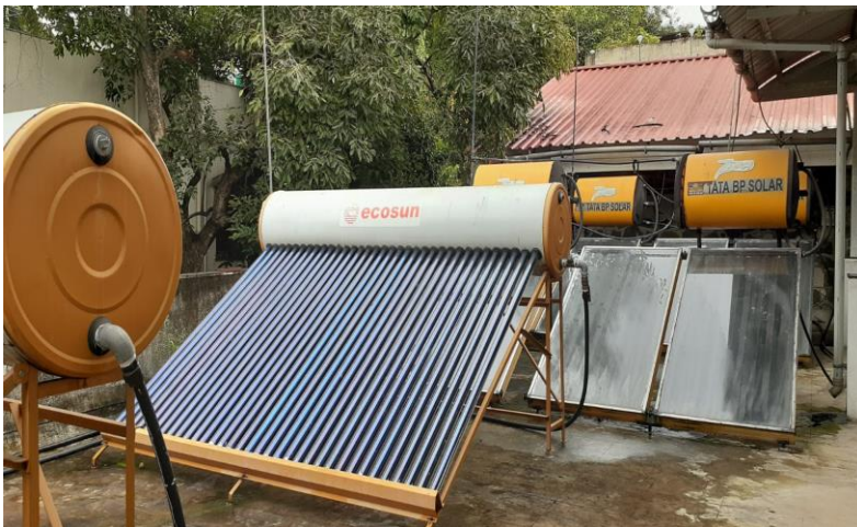
SOLAR PANELS for Electricity , Pragnyalaya , Pune
