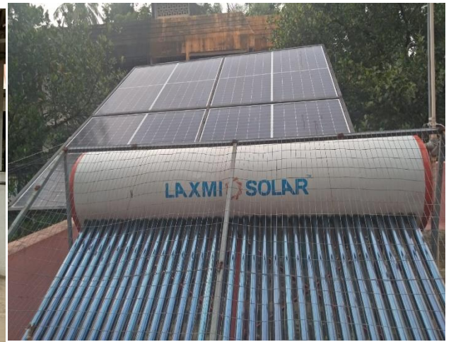
SOLAR PANELS for Electricity and water heating, Ashadeep , Malvan
